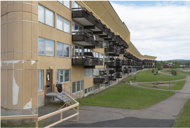
Figure 6. Ralph Erskine. Ormen Långe, Svappavaara, 1963–65. View of the southern façade, 2006. RAÄ 160010000093302. Photo: Bengt A Lundberg.
